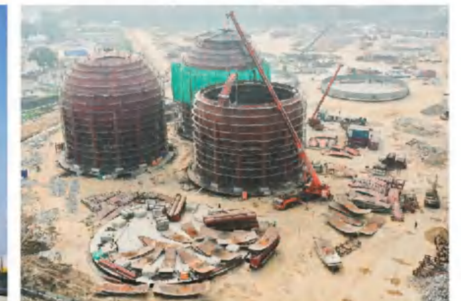
Nigeria 4x10000m 3 Spherical Tanks
