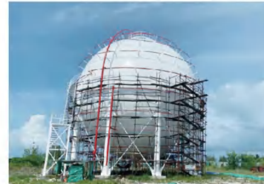
Maldives 3000m 3 Spherical Tank
